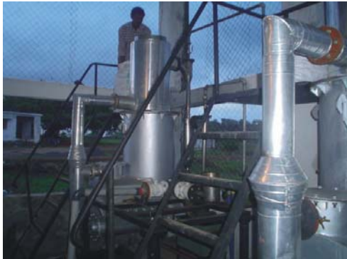
2 x 10 kWe Gasifier System at Kasai
